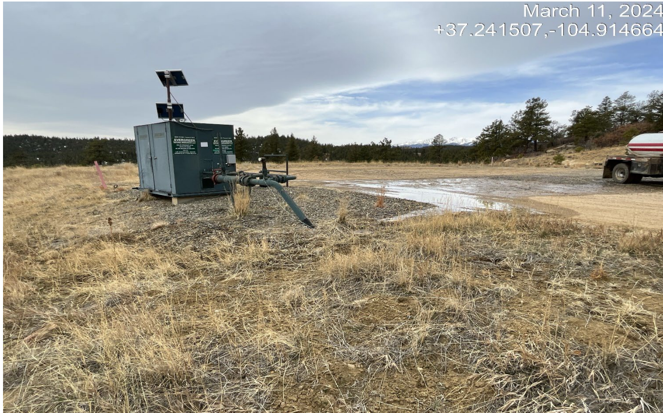
Photo 1. Facing southwest toward the location. There was water from a leak that spread across the location from right to left side of photo.
