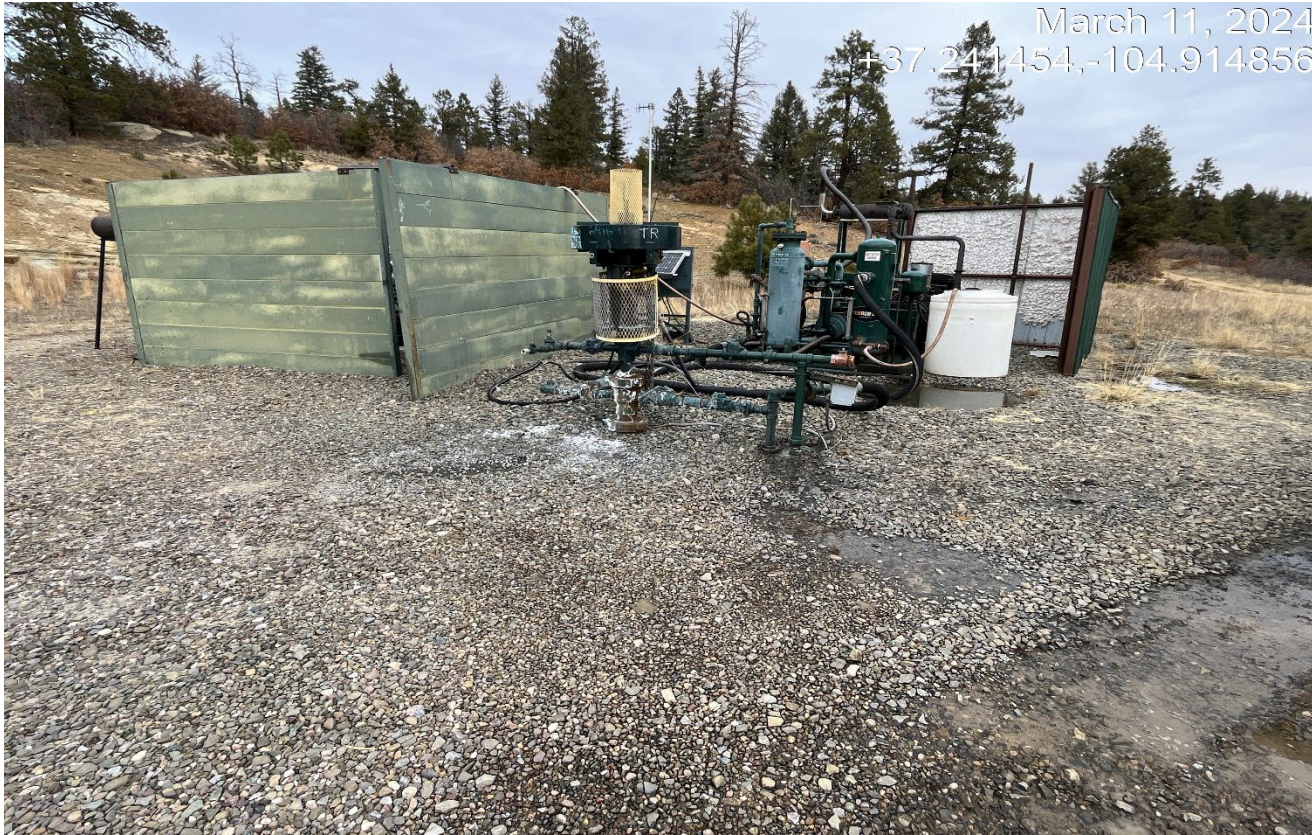
Photo 2. Facing toward the wellhead.
