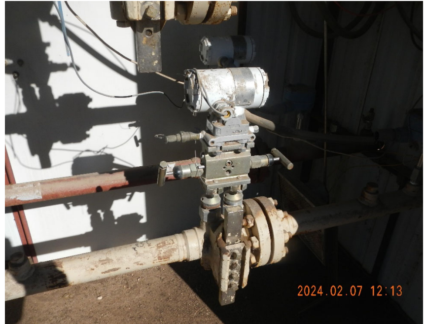
6. Digital gas meter inside meter shed.
