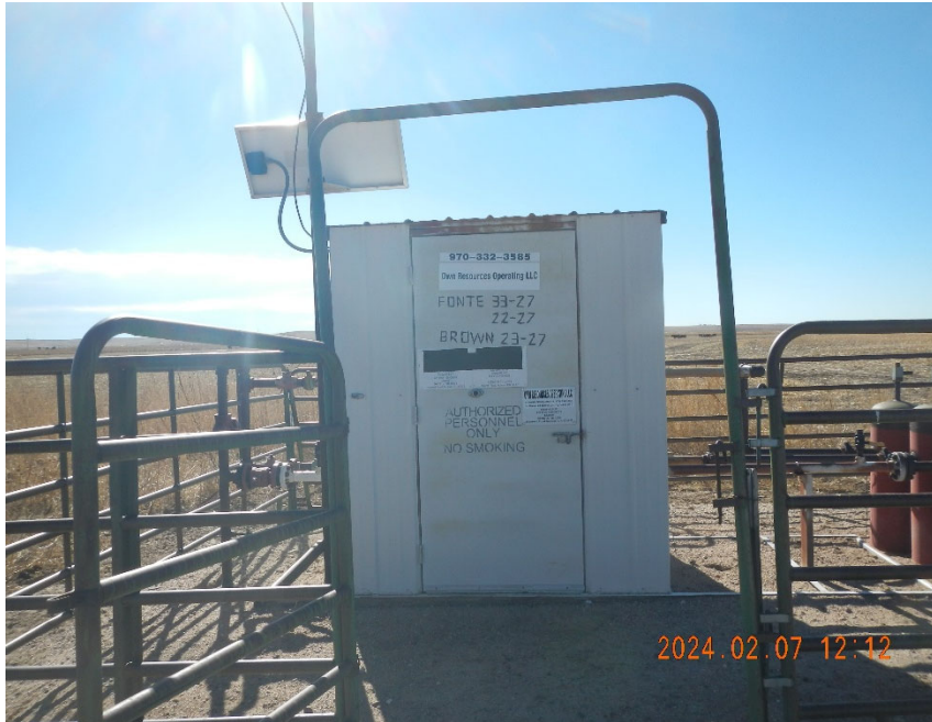
5. Shared remote gas meter shed at remote gathering location.
