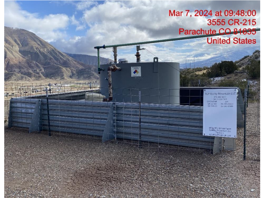
Tank Battery – Photo #09725
