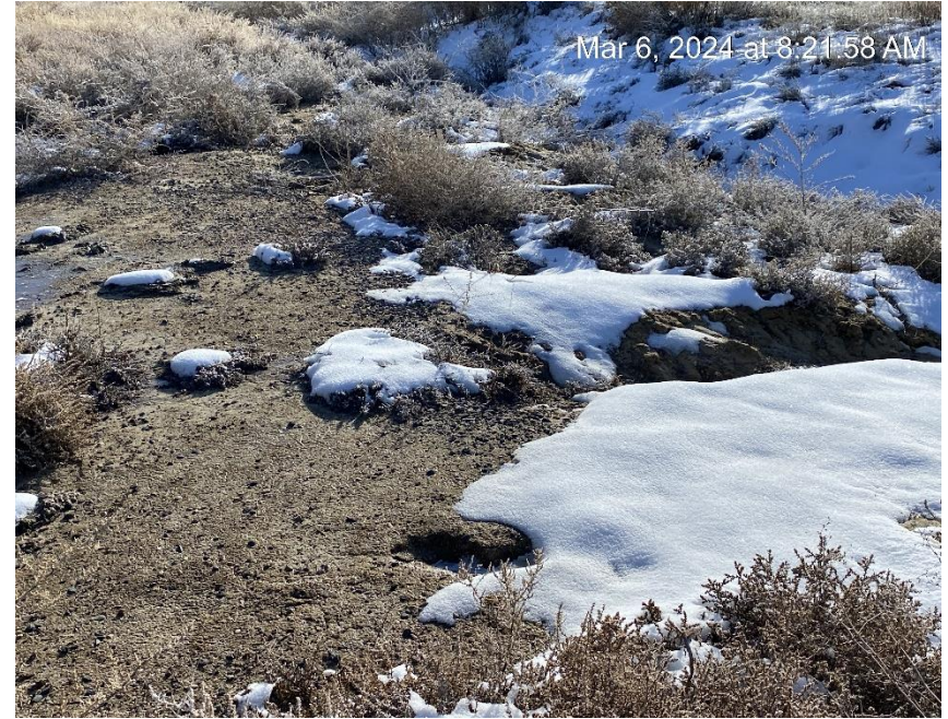
Erosion and sediment migration
