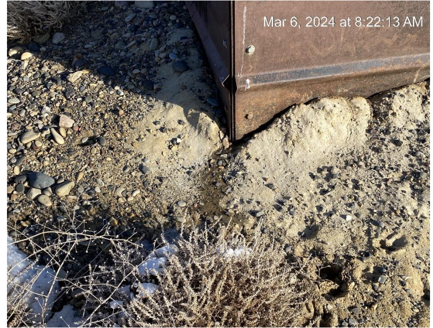
Containment still leaking from 4/11/23 inspection
