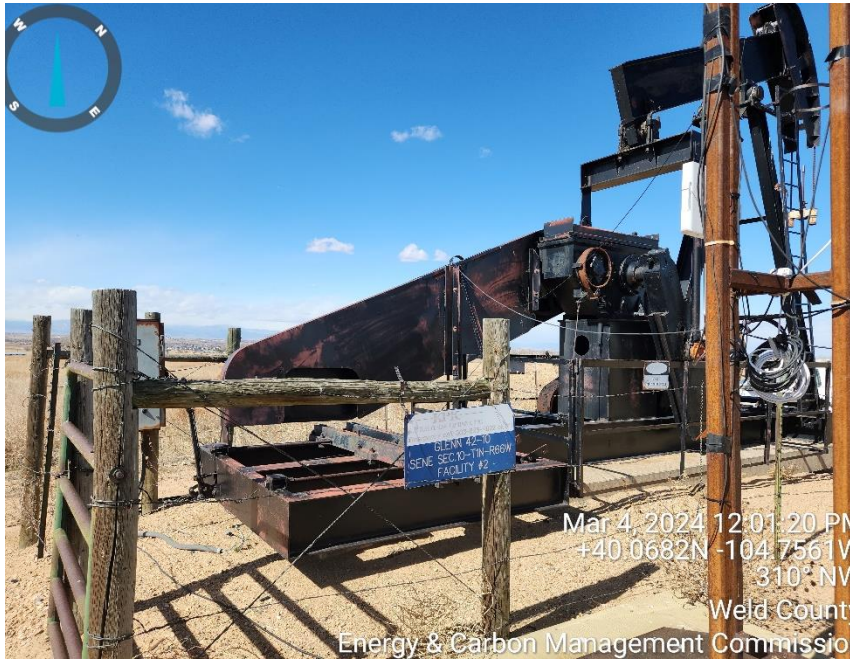
Photo 3 pumping unit and equipment
