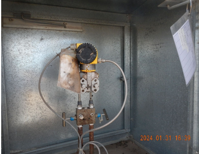
3. View of digital gas meter inside meter box.
