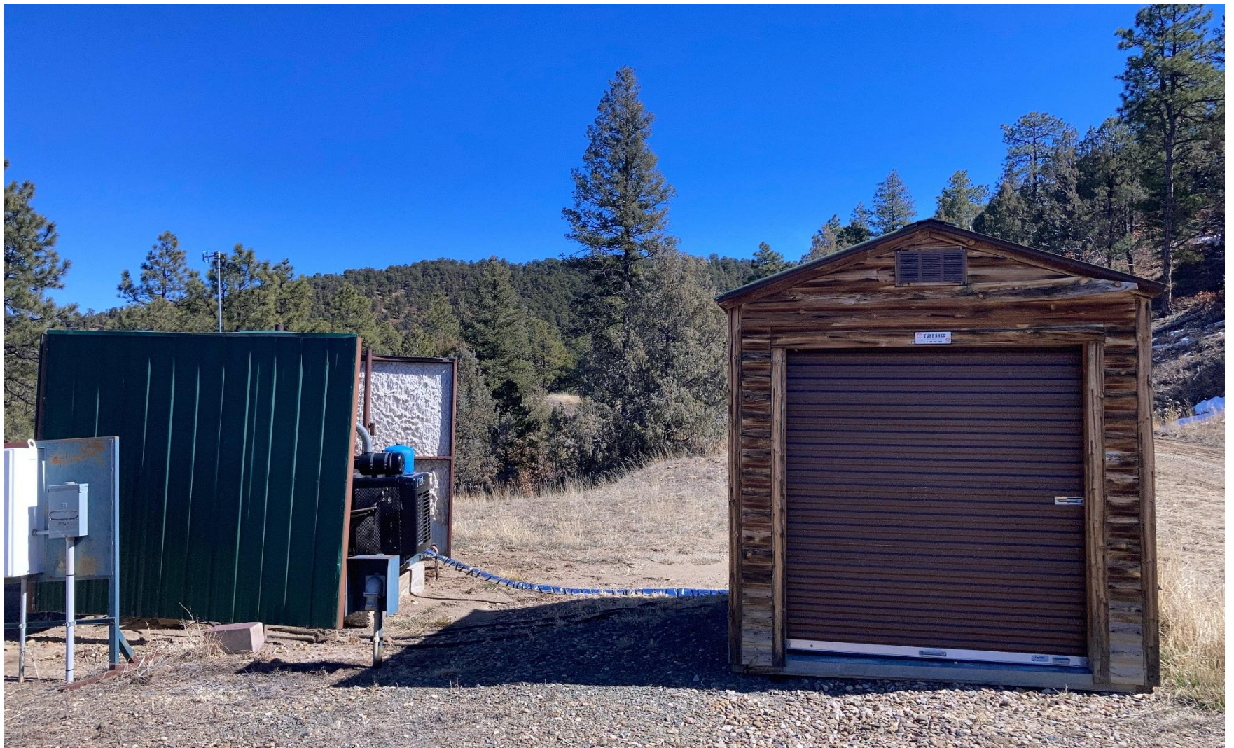
PHOTO 3: WELLHEAD AND EQUIPMENT
