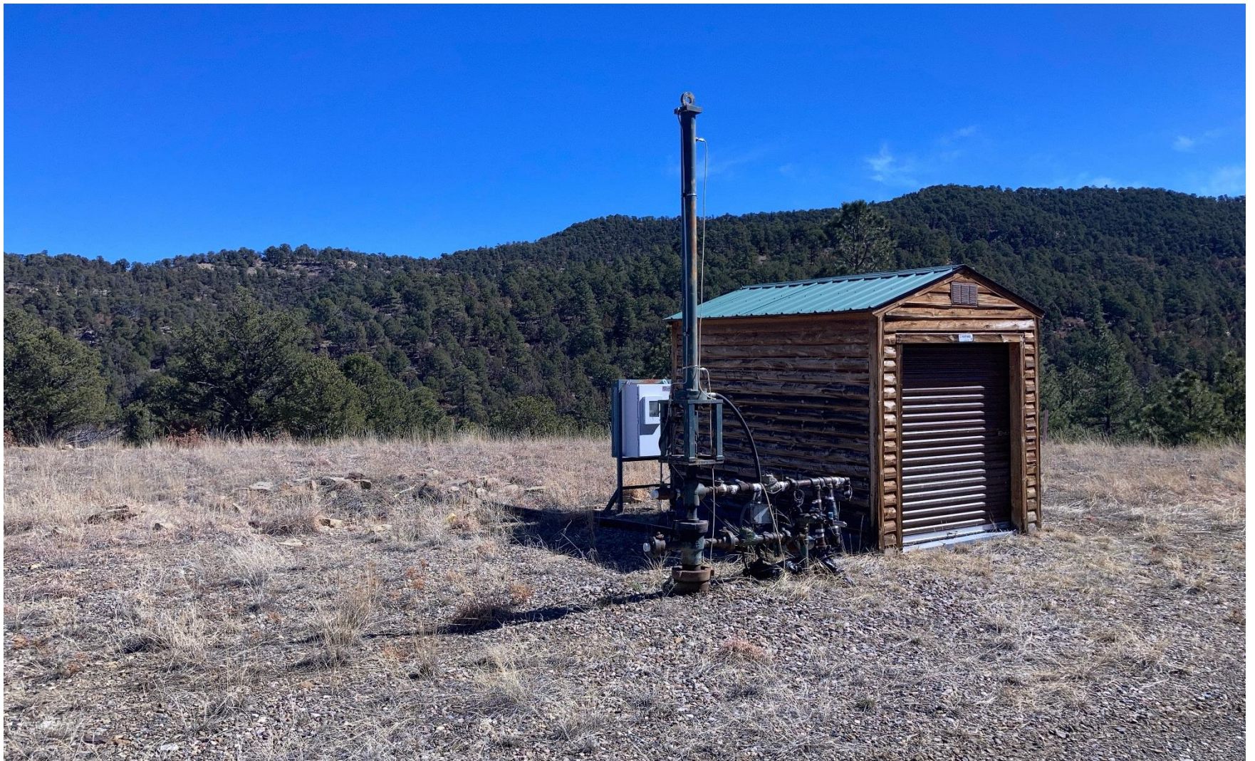
PHOTO 3: WELLHEAD AND EQUIPMENT
