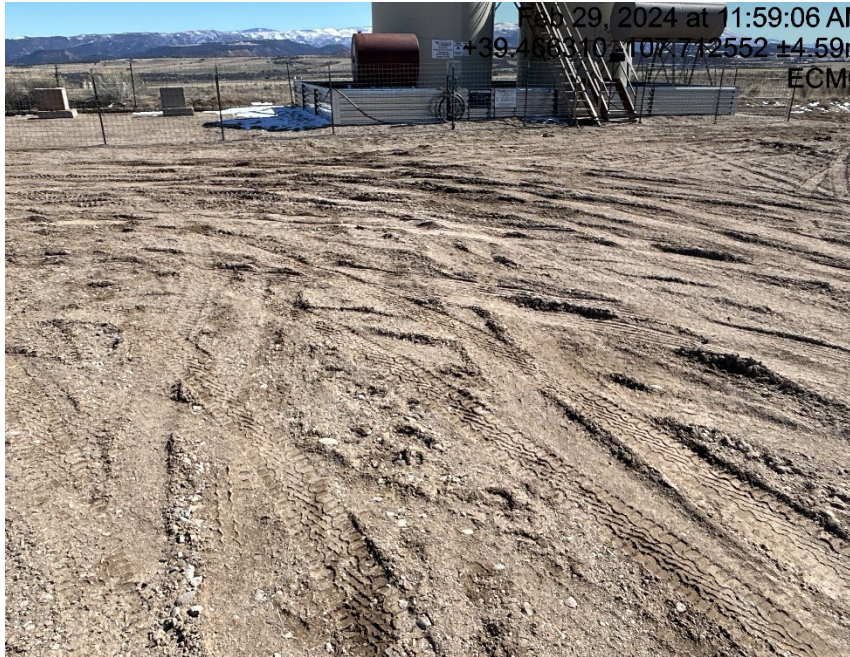
Lack of stabilization
