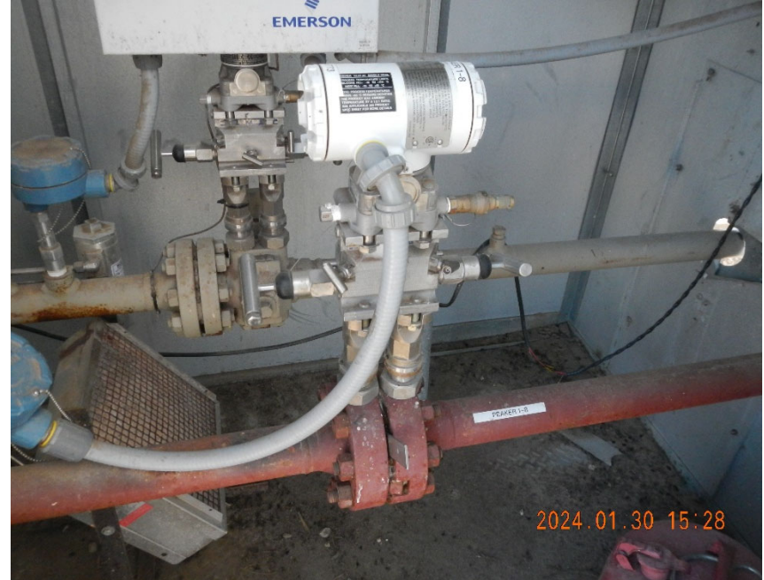
6. Digital gas meter inside meter shed.
