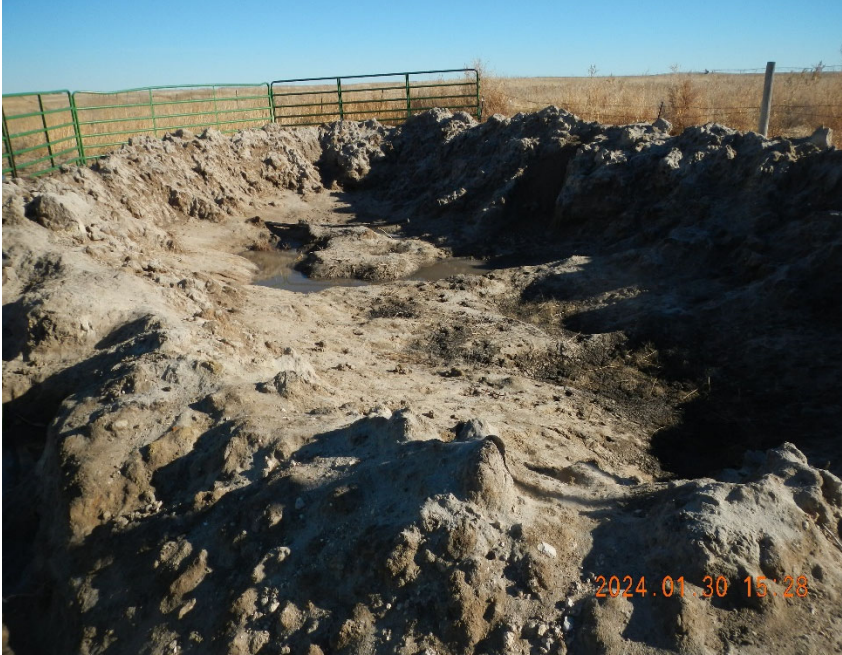
7. View of produced water pit. Berms need dressing.
