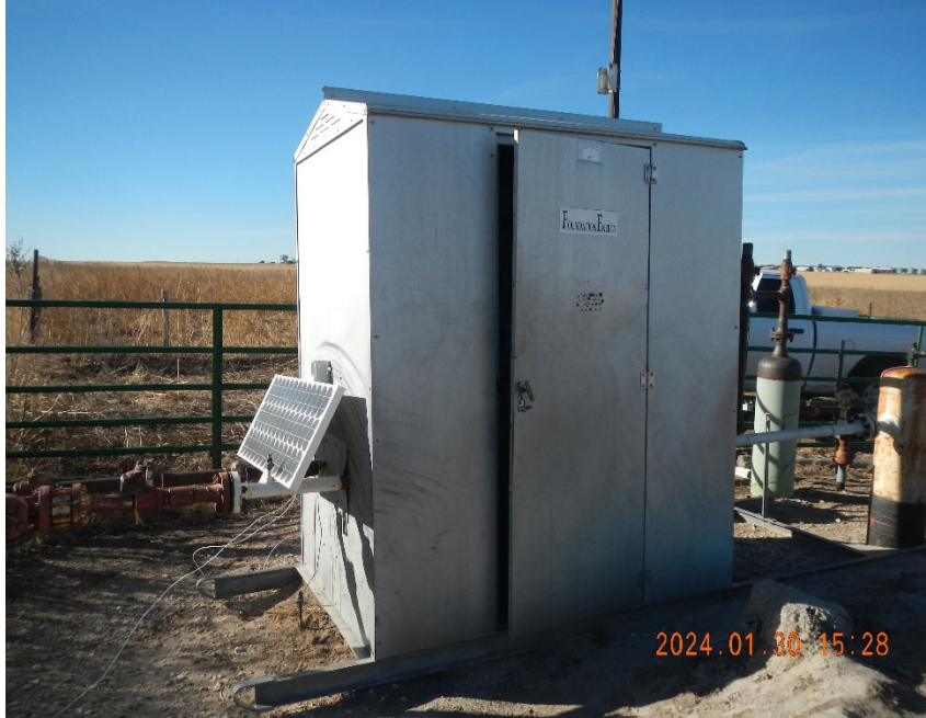
5. Shared remote gas meter shed.
