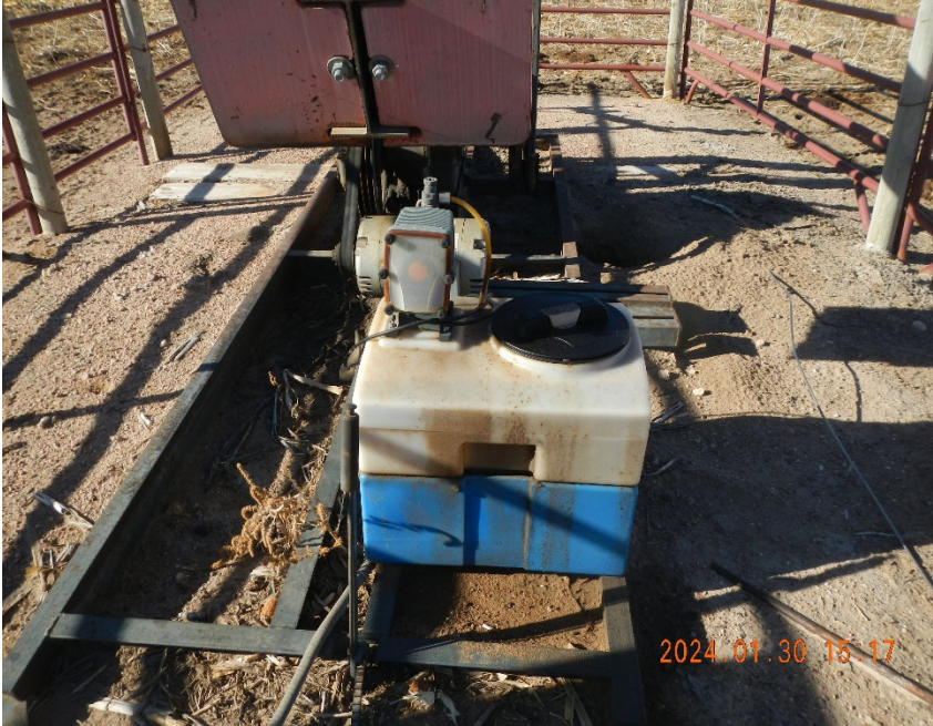
3. Chemical tank and injection pump. Currently not in use. No label.
