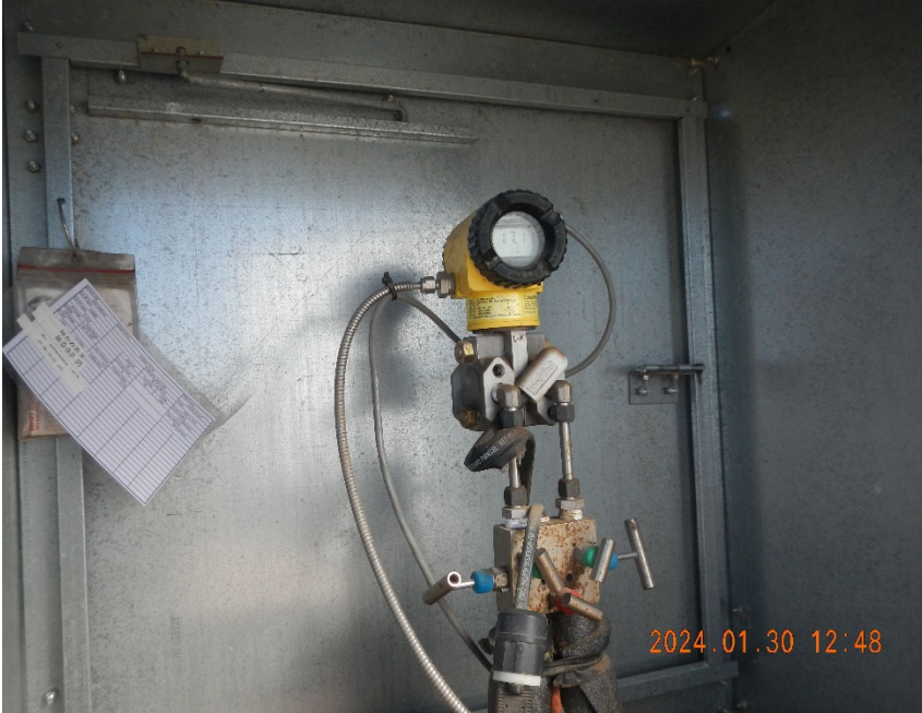
3. Digital gas meter inside meter box.
