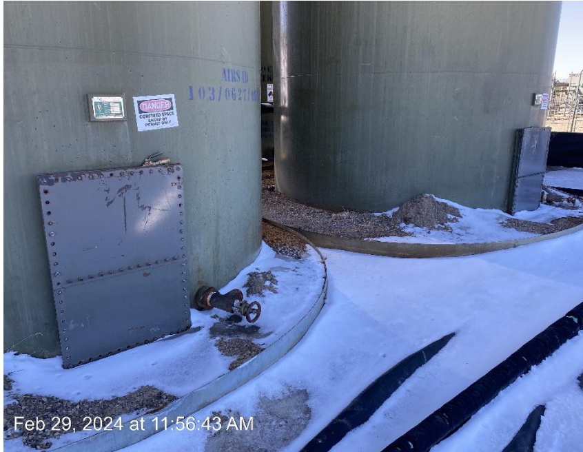
Tanks out of service
