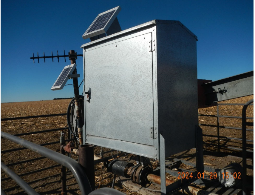
3. Flowline mounted gas meter run box.
