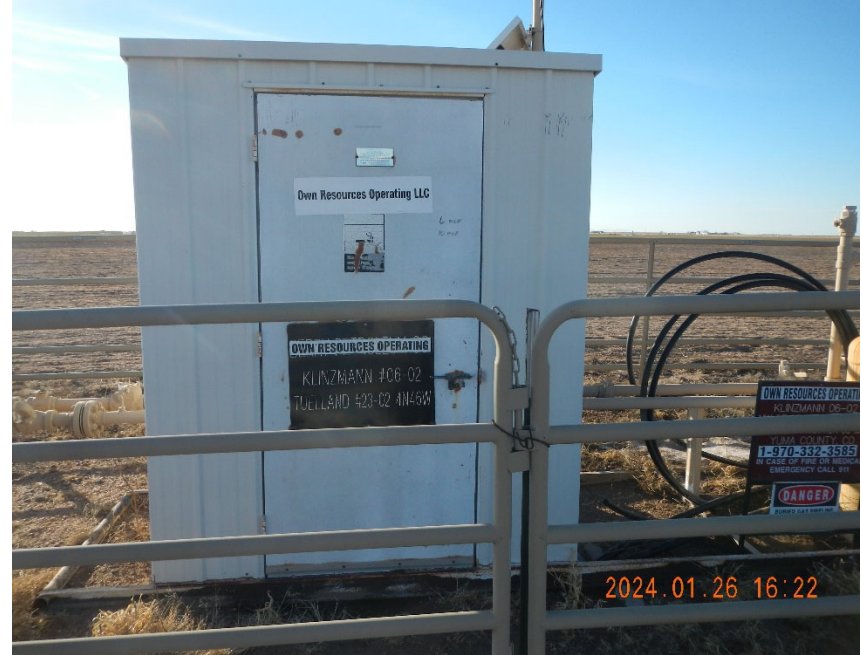
4. Shared gas meter run shed.
