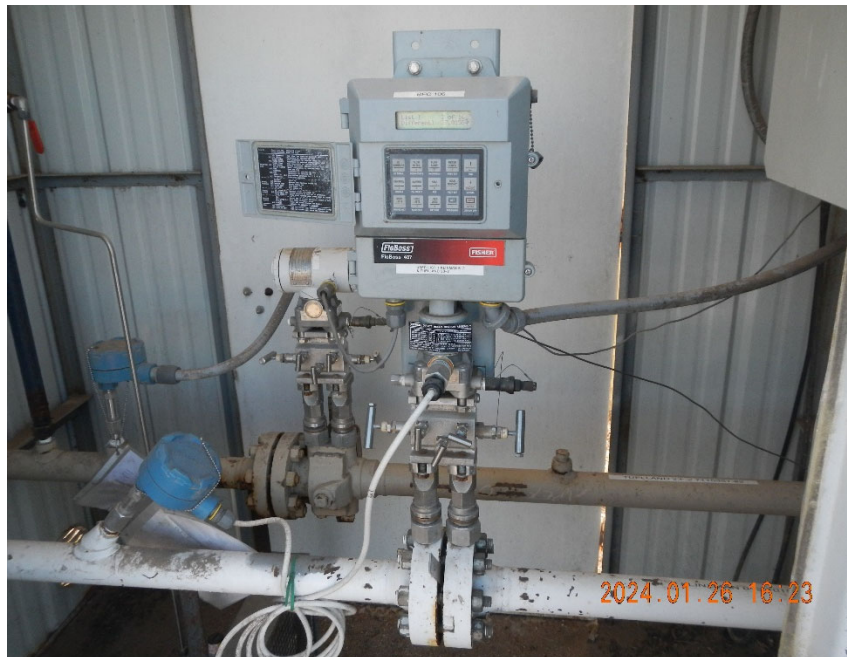
5. Gas meter inside meter shed.
