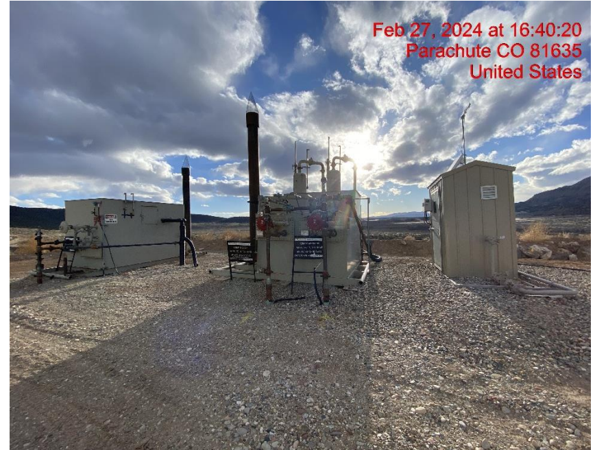
Separators/Gas Meters – Photo #09622
