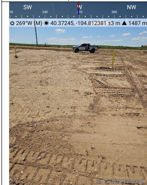
Looking West at tank battery and separator location – 40.372450 / -104.812381
