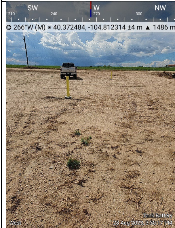
Looking West at tank battery and separator location – 40.372484 / -104.812314
