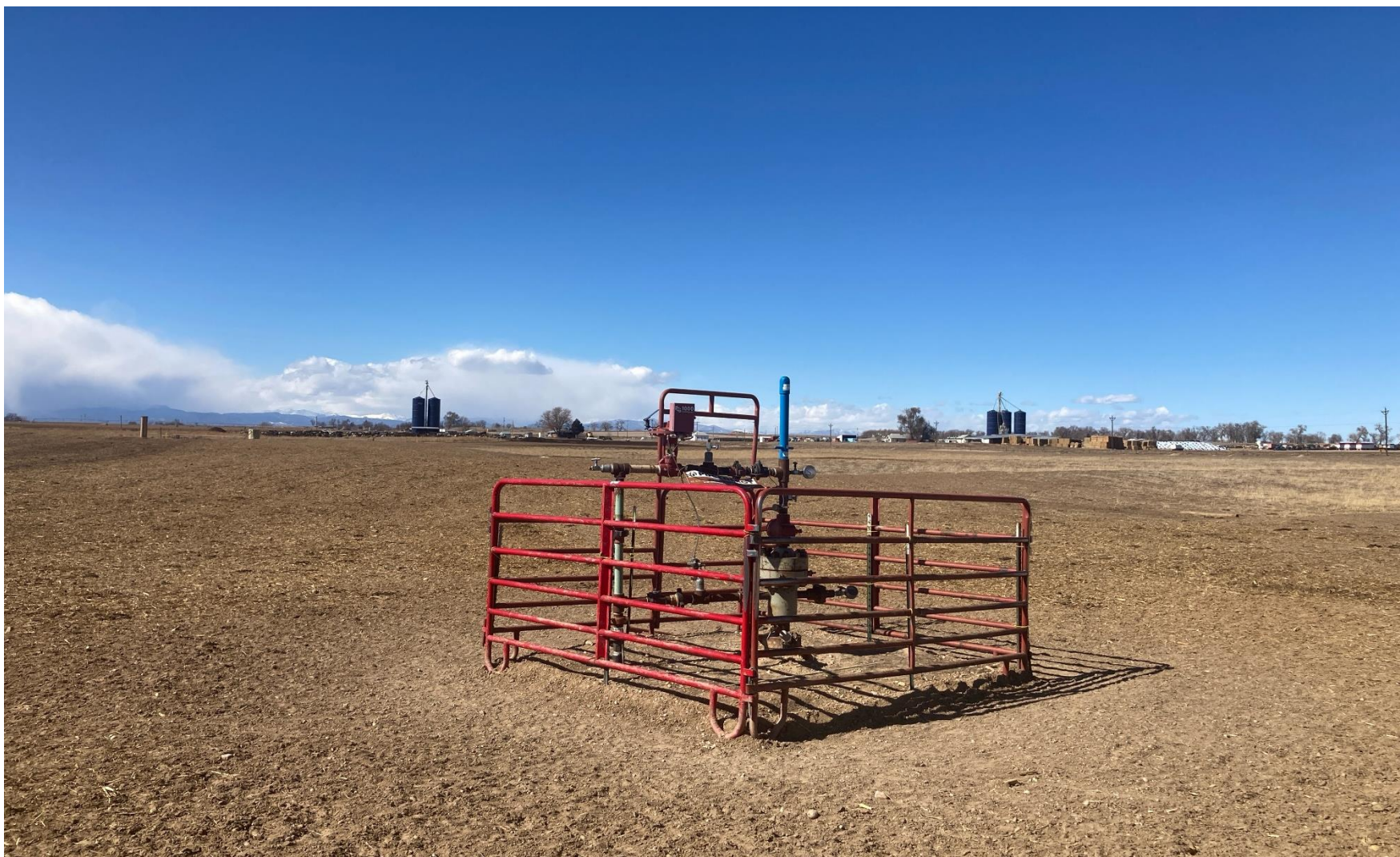
PHOTO 3: WELLHEAD AND EQUIPMENT
