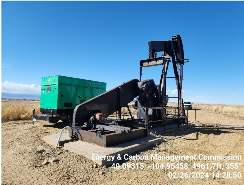
Photo 5 Pump Jack & Free standing mobile generator.
