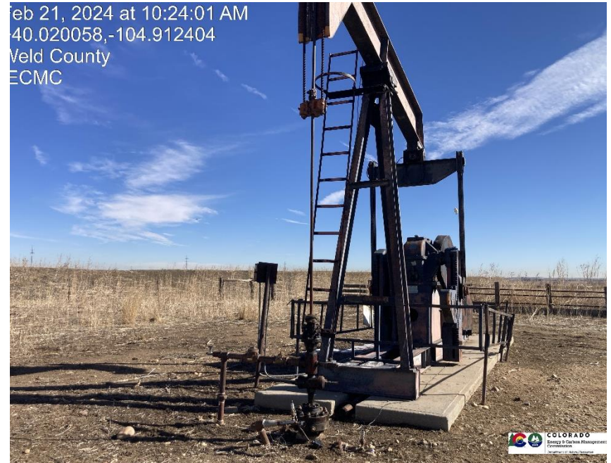
Pic 2 pump jack / wellhead
