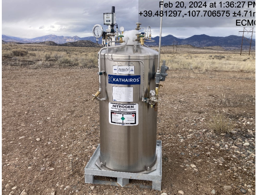
Nitrogen running pneumatic devices.
