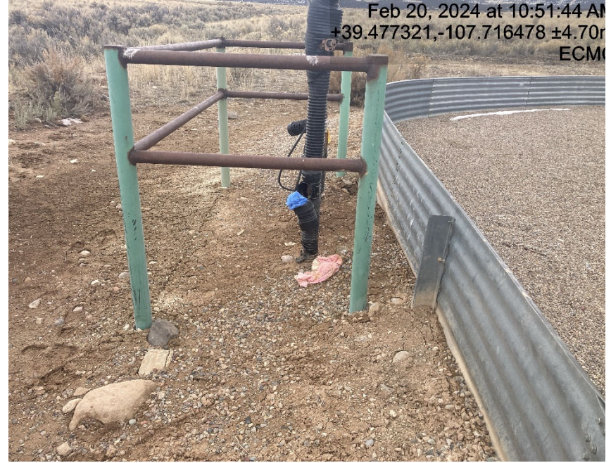
Debris and open pipeing
