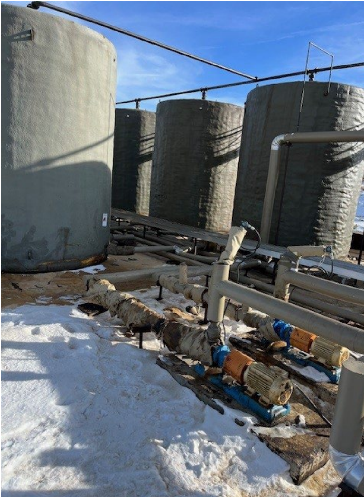
PHOTO NO 6: SPILL AREA IN NW CORNER OF CONTAINMENT LOOKING SE
