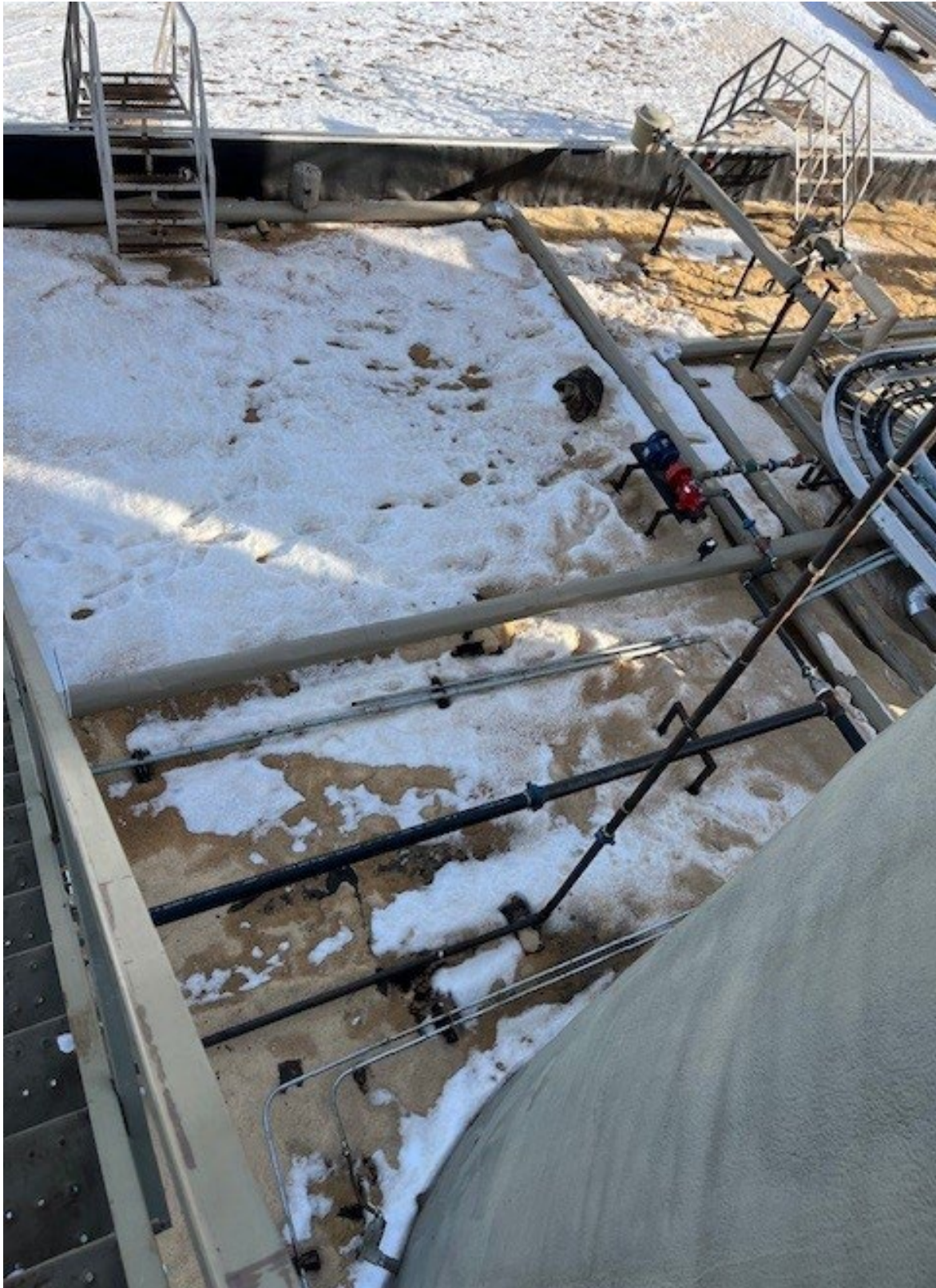
PHOTO NO 4: SPILL AREA FROM NE MOST TANK LOOKING INTO NE CORNER OF CONTAINMENT
