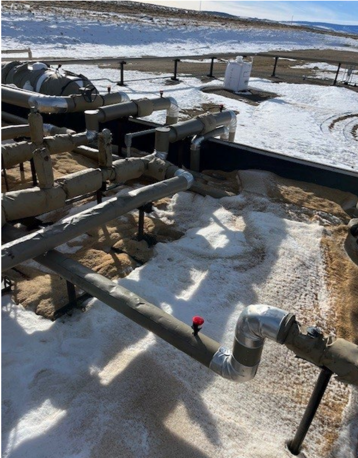
PHOTO NO 8: SPILL AREA LOOKING SW FROM NW CORNER OF CONTAINMENT
