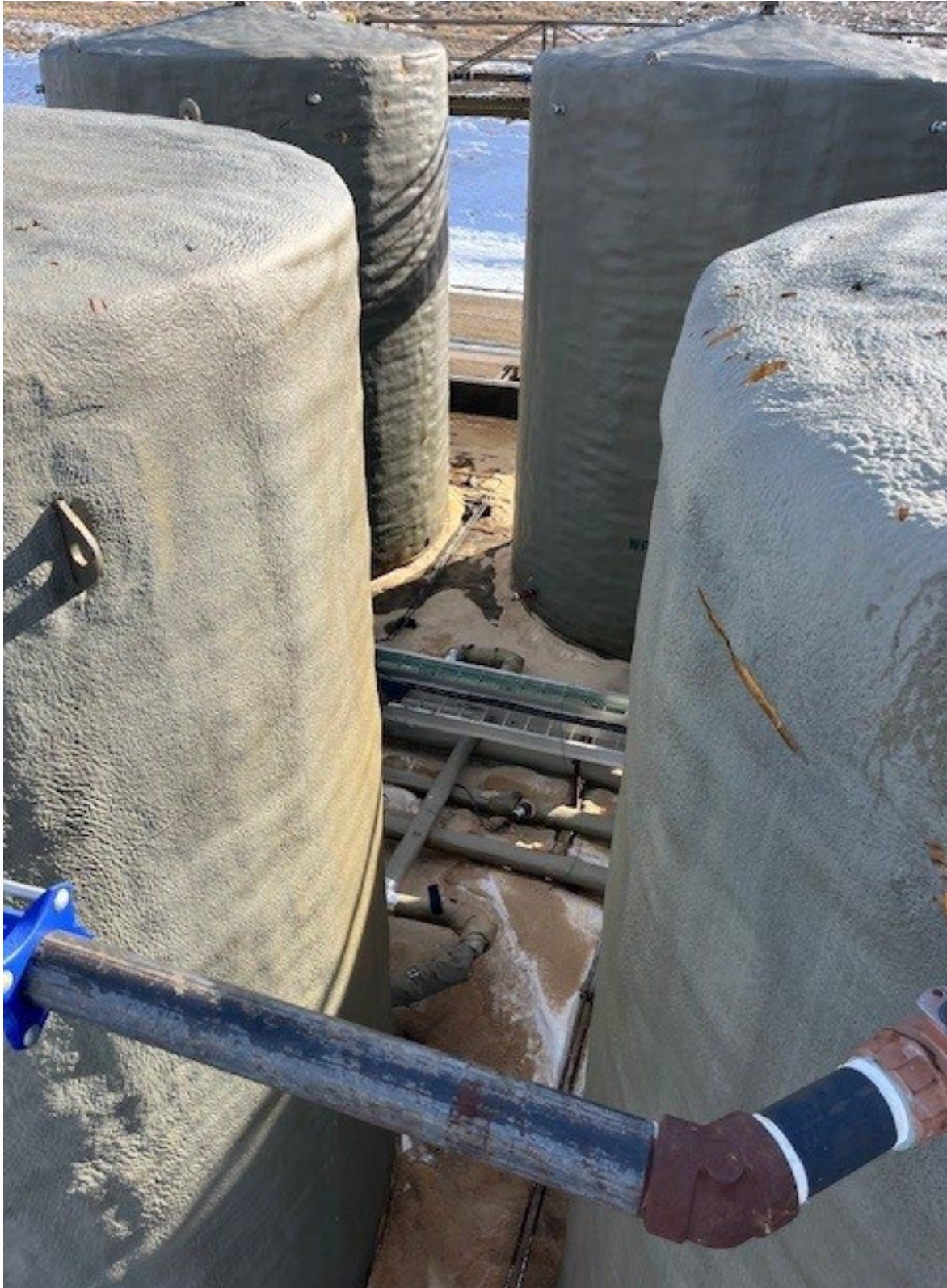
PHOTO NO 3: SPILL AREA BETWEEN TANKS LOOKING SOUTH
