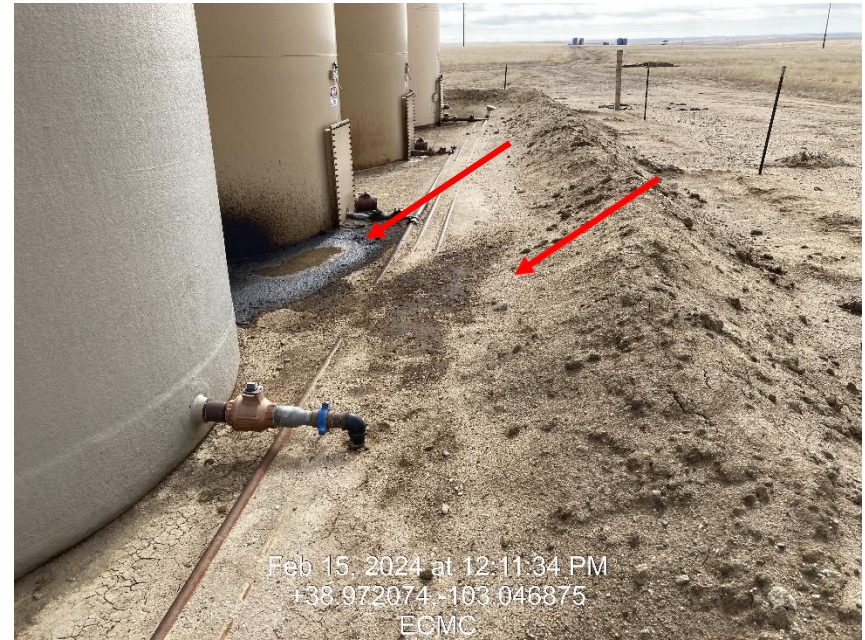
Photo 2 – Impacted Soils at Tank Battery
