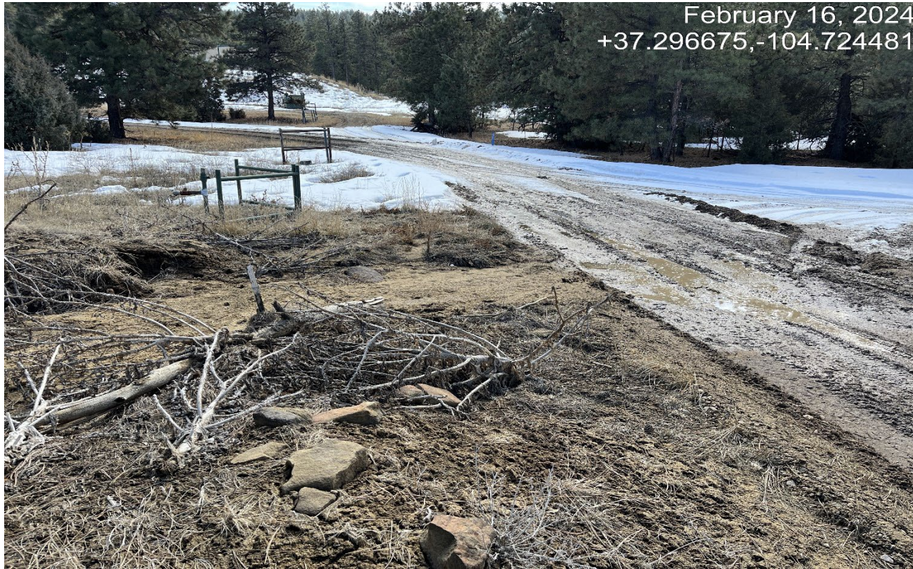
Photo 1. Facing southeast along the access road . This culvert is filled in with sediment causing erosion of the road..
