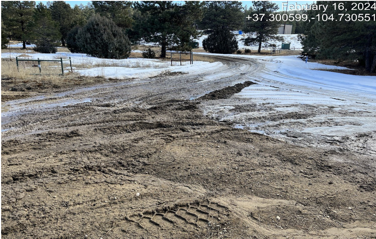
Photo 2. There is erosion across the road at the intersection where culvert is plugged.,
