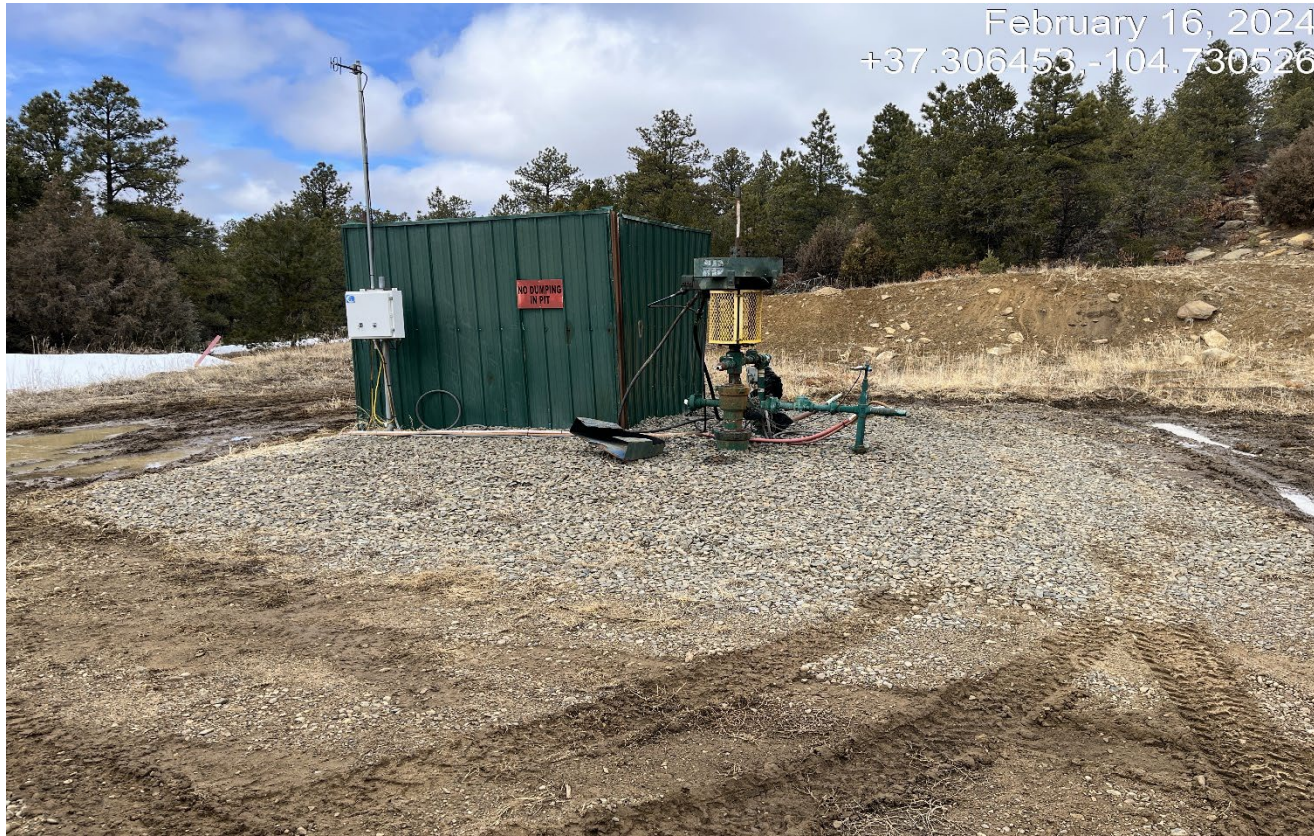
Photo 4. Facing toward the wellhead.
