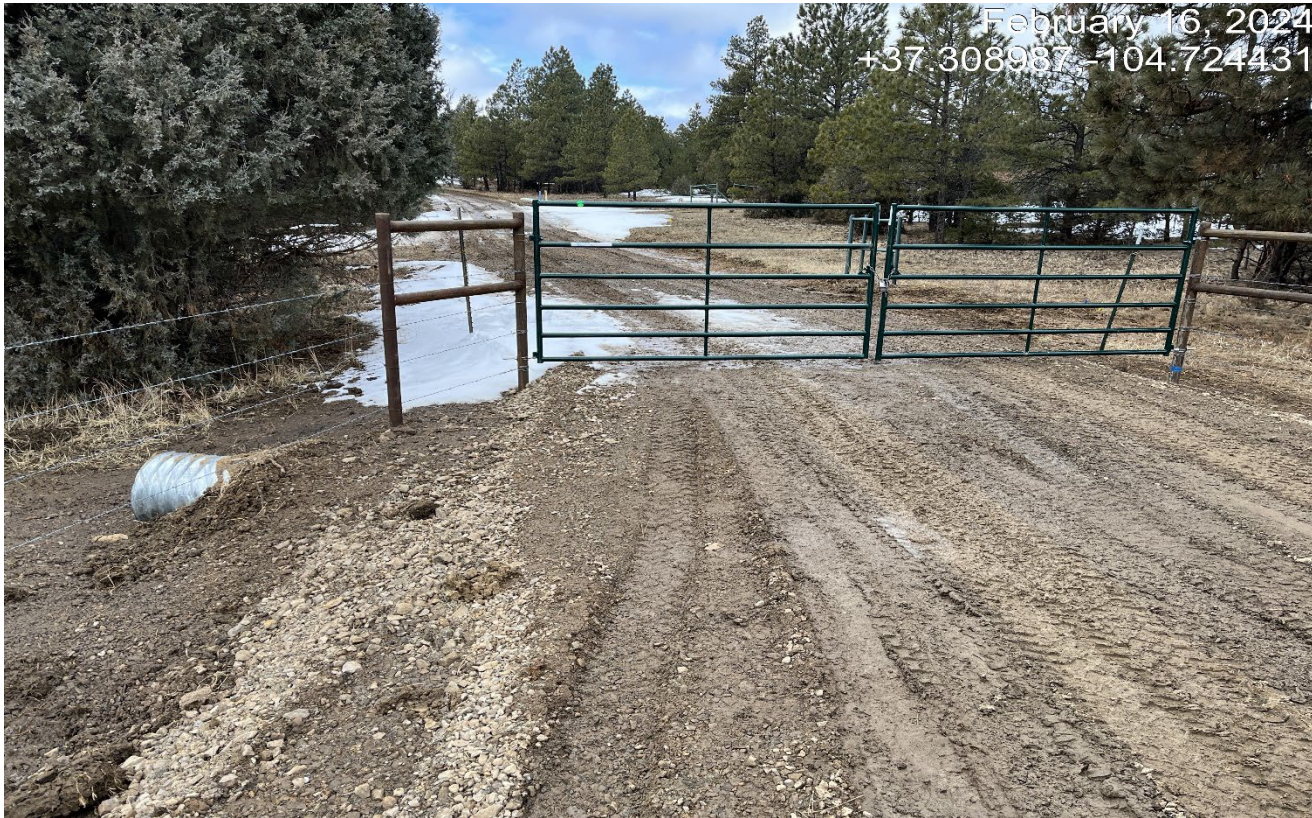
Photo 1. Facing west at beginning of the road. It appears a new culvert was installed at this area.
