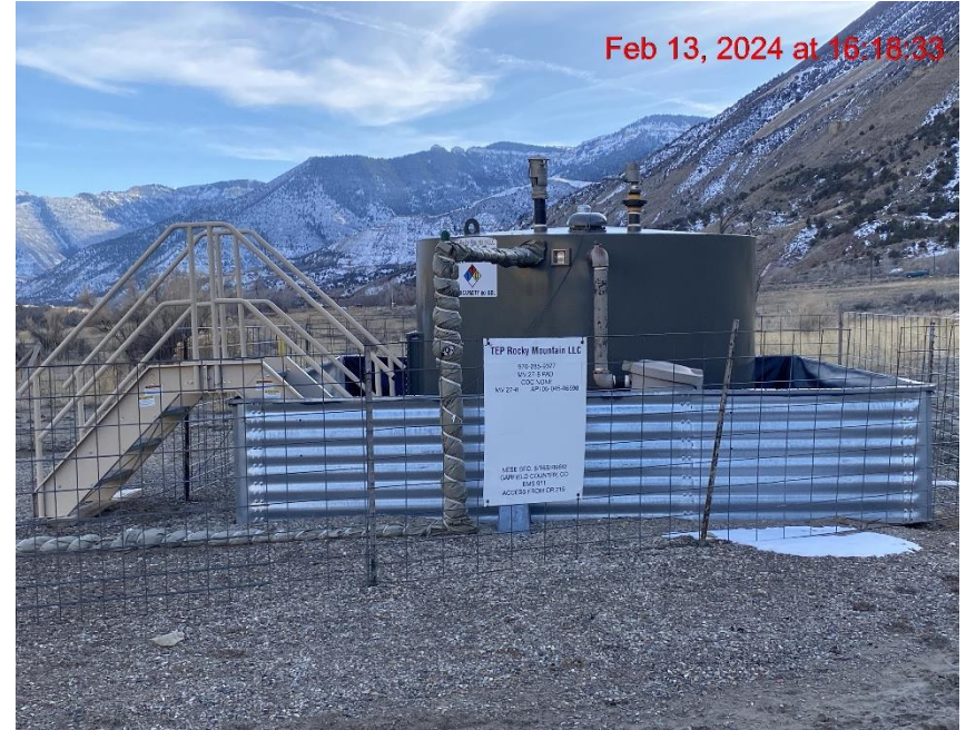
Tank Battery – Photo #09305
