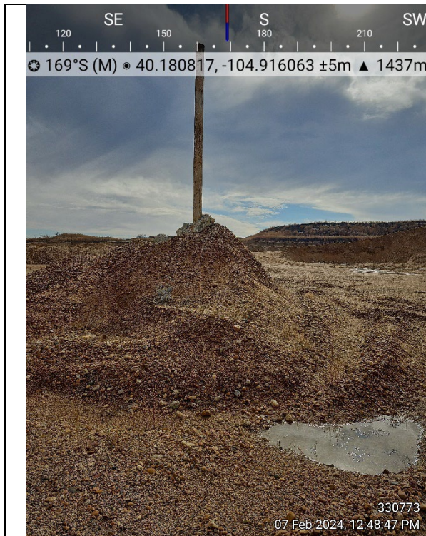
Looking South at Nelson 23-32 well pipe – 40.180817 / -104.916063
