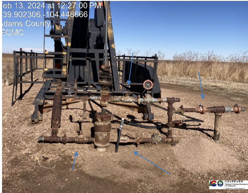
Pic 3 flowlines appear to be open.
