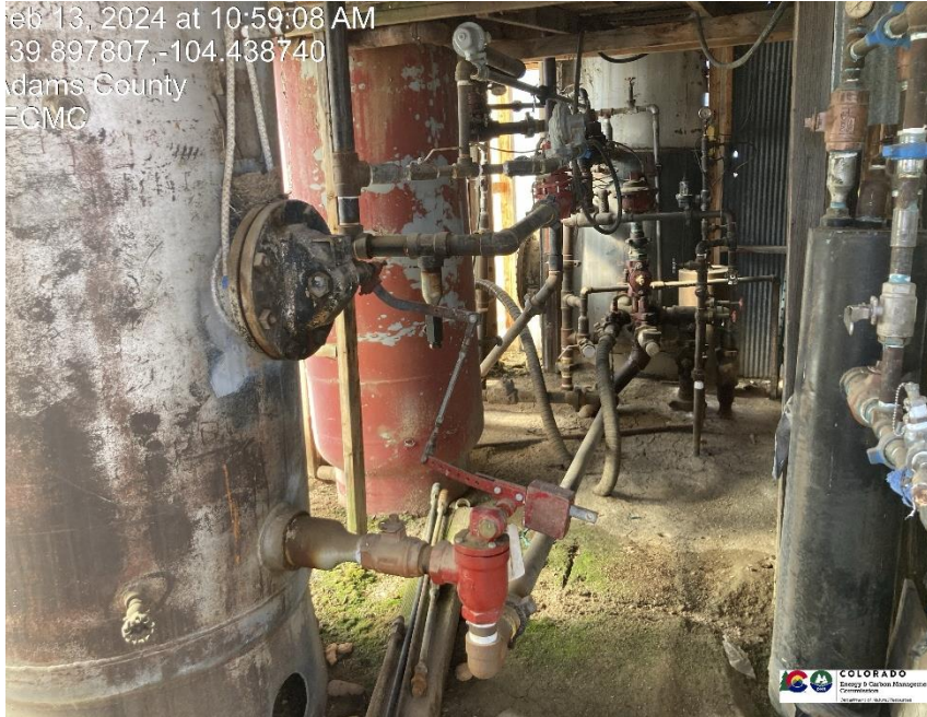
Pic 5 Separator house
