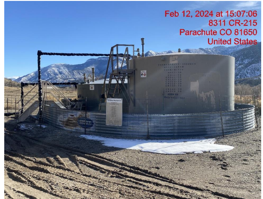
Tank Battery – Photo #09240
