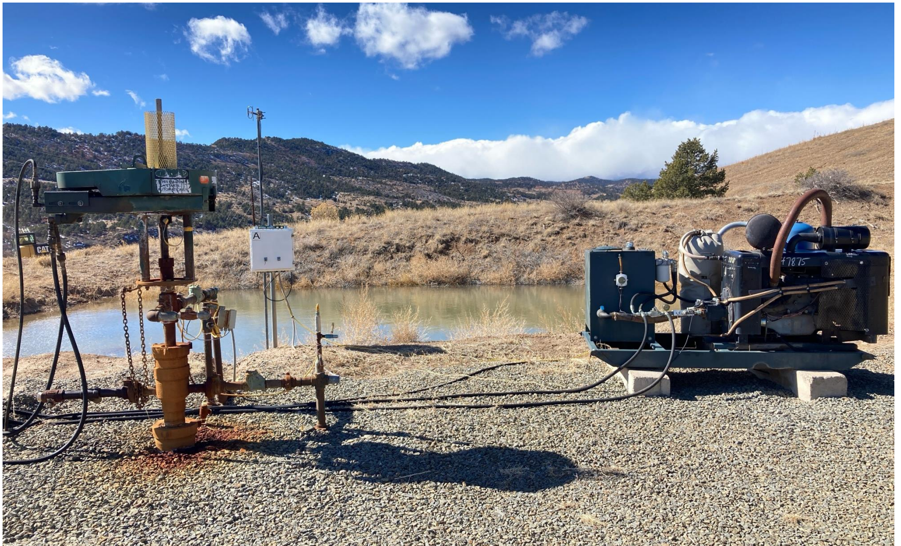
PHOTO 3: WELLHEAD AND EQUIPMENT
