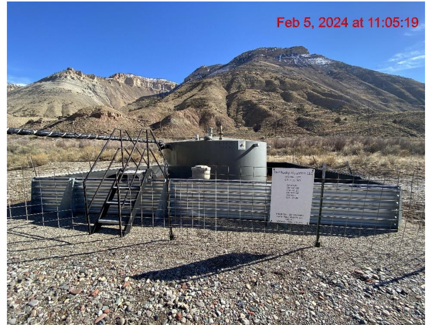
Tank Battery – Photo #09147
