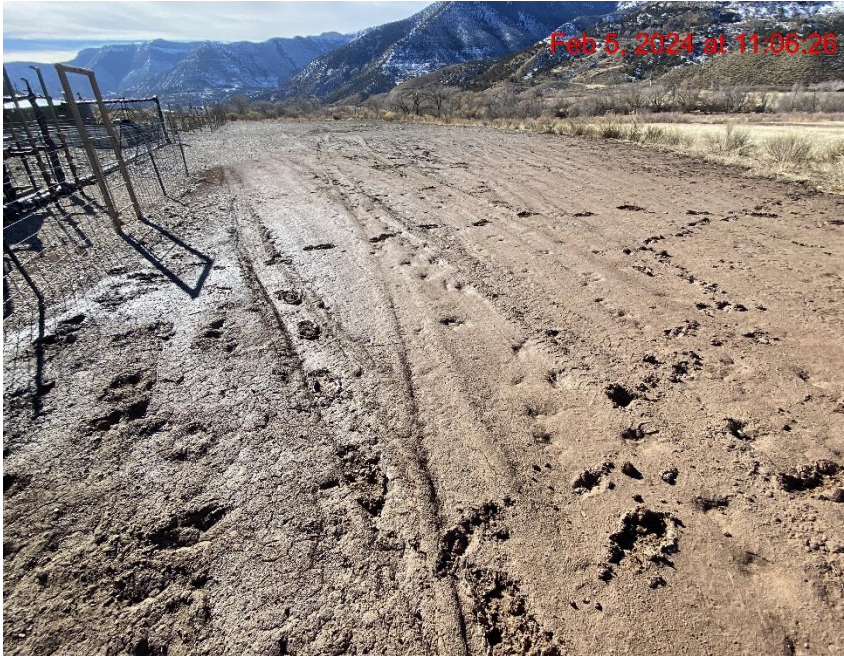
Lack of Stabilization – Photo #09150
