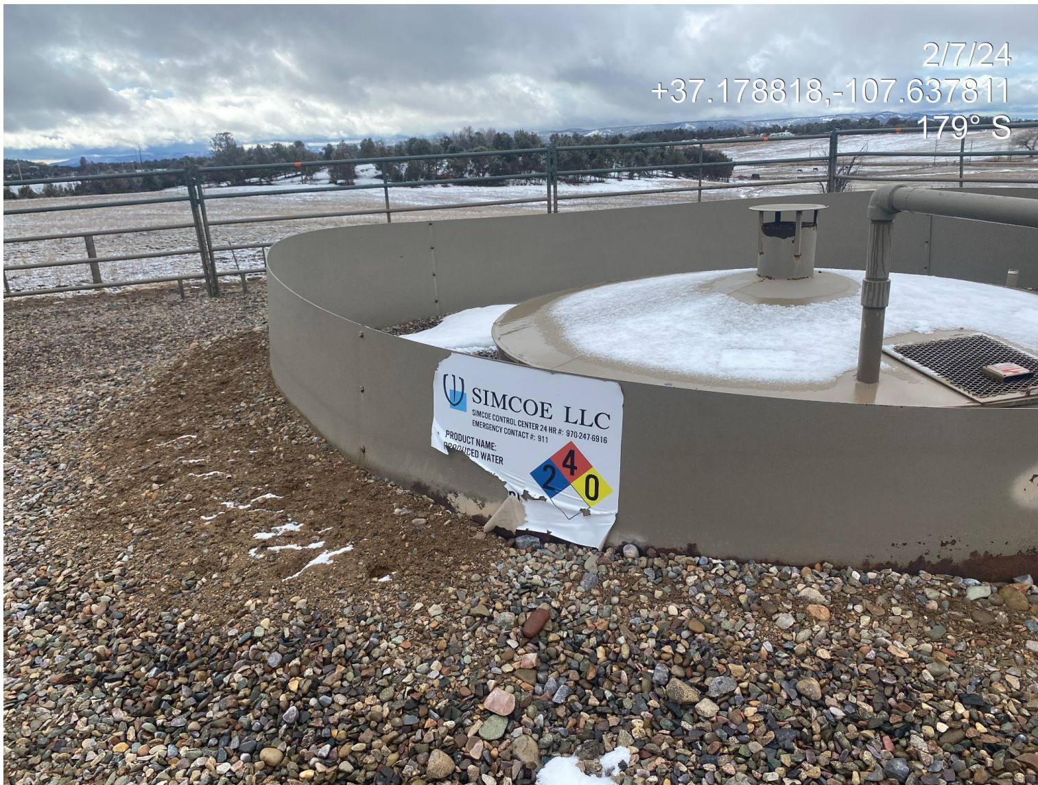
Photo 4. View of deteriorating produced water sign on location.
