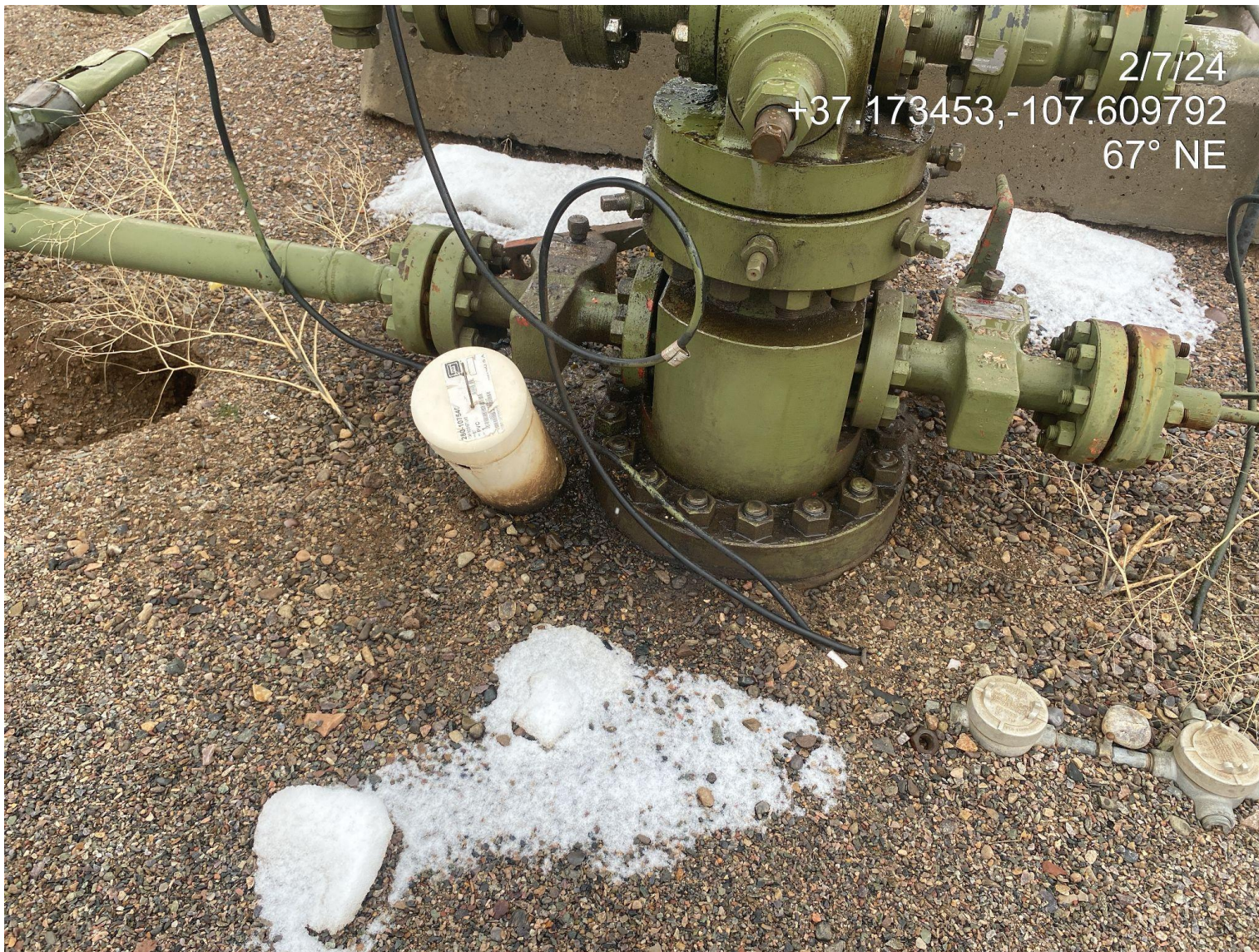
Photo 4. Impacted soils observed at the well head.
