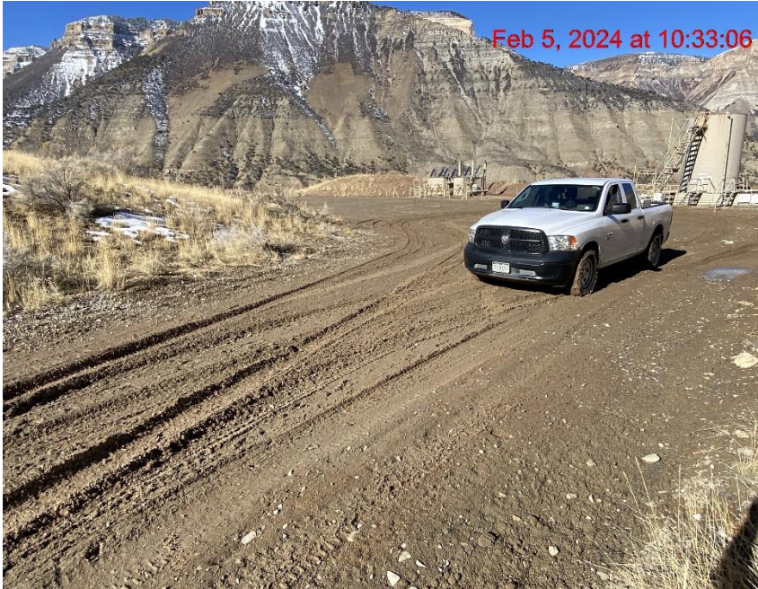
Insufficient Vehicle Tracking BMPs at Location Entrance/Exit – Photo #09118
