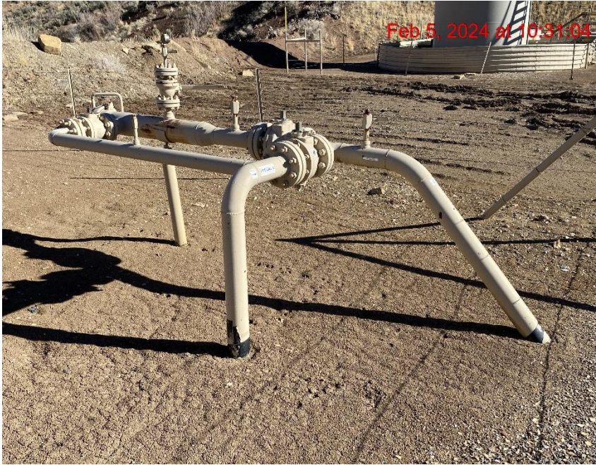
Pig Station – Photo #09113
