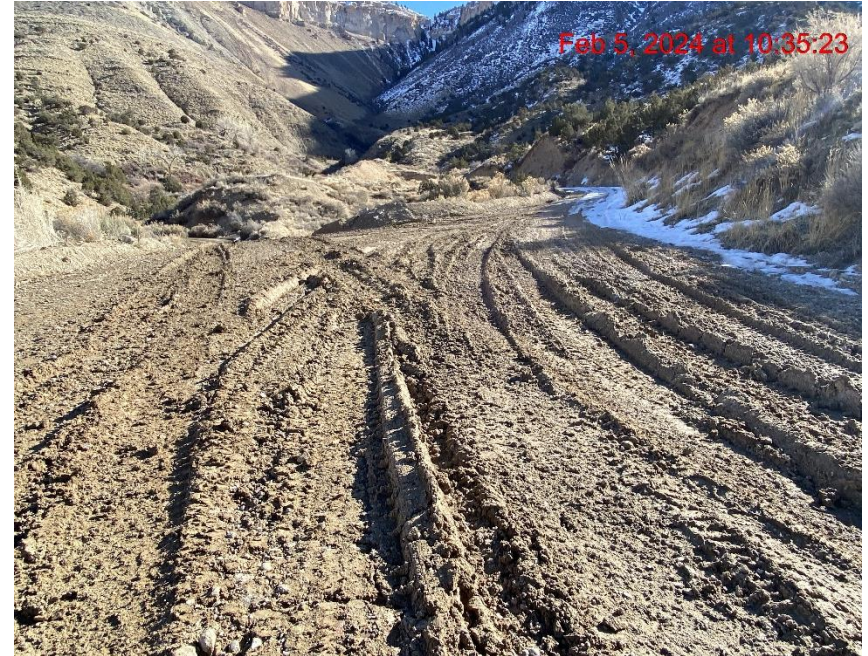
Lease Road Lacks Stabilization – Photo #09119
