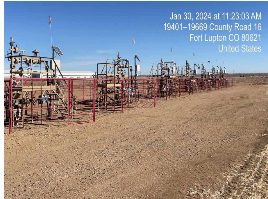
Photo 2. Photo taken of well heads. Photo taken facing northeast.
