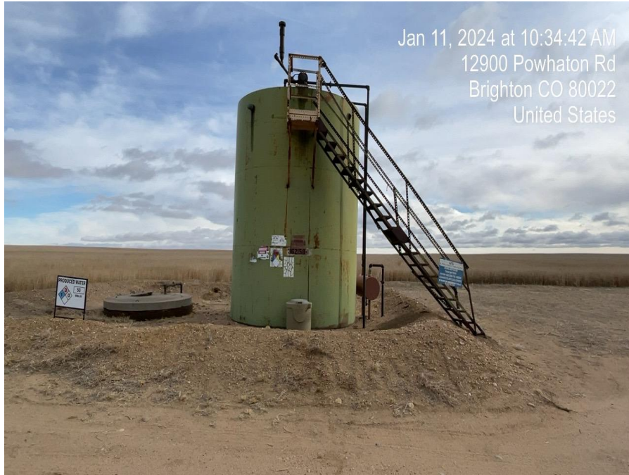
Photo 3. Photo taken of tank battery. Photo taken facing southeast.
