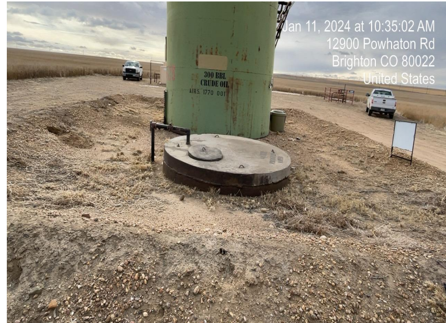
Photo 6. Photo taken of tank battery/buried tank and mowed vegetation. Photo taken facing northwest.
