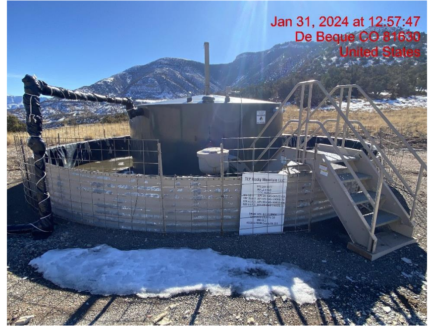
Tank Battery – Photo #09037
