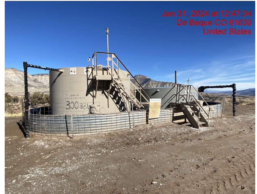
Tank Battery – Photo #09025
