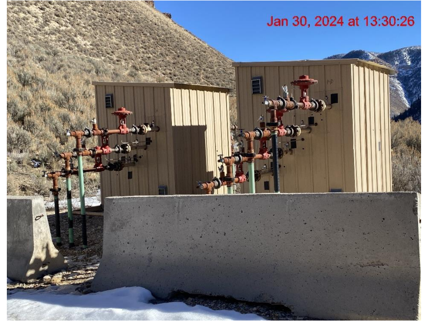
Gas Lift – Photo #09002
