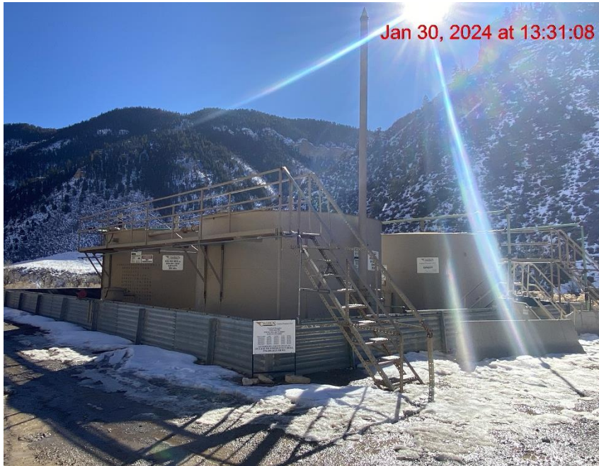
Tank Battery – Photo #09004
