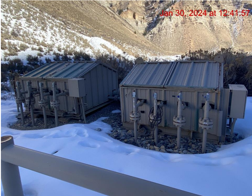
Gas Meters – Photo #08941
