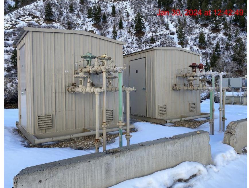
Gas Lift – Photo #08945
