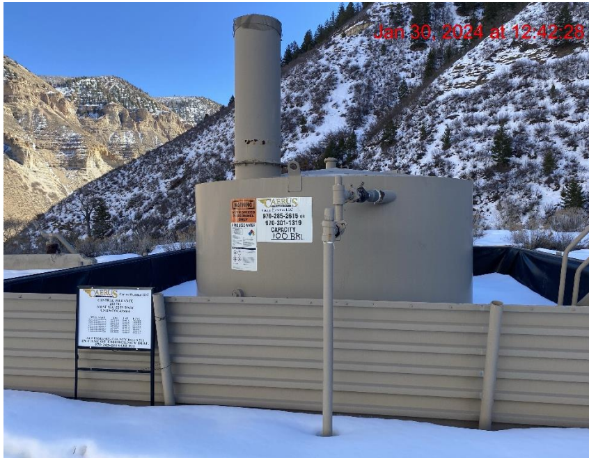
Tank Battery – Photo #08943
