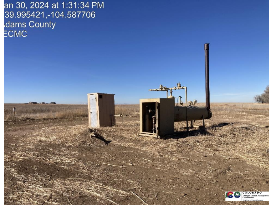
Pic 2 Separator, GMR
