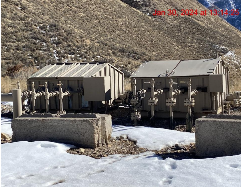
Gas Meters – Photo #08983
