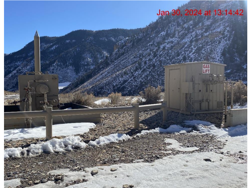
Separator/Gas Lift – Photo #08984
