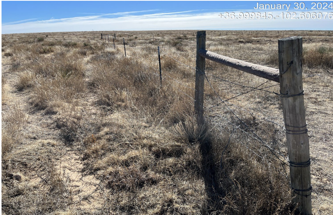
Photo 3. There is a perimeter fence that remains in disrepair around the location.
