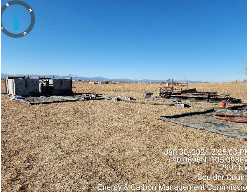
Photo 1 well servicing equipment
