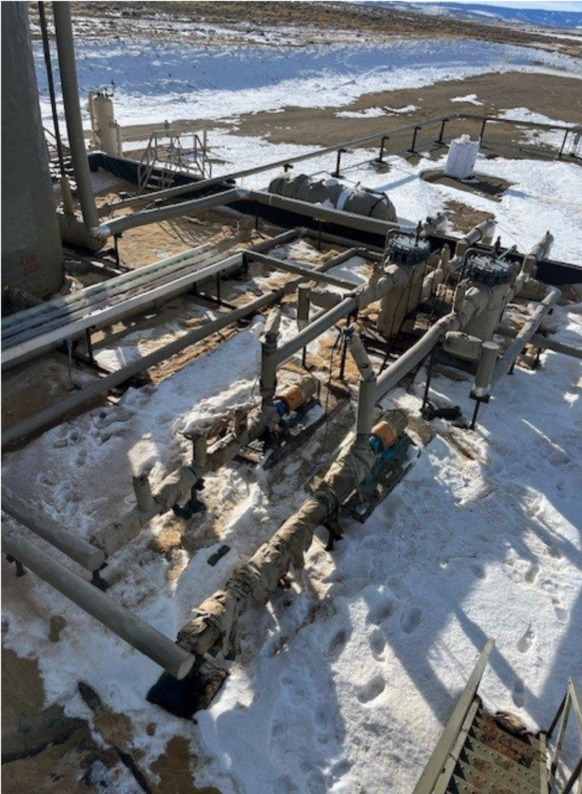
PHOTO NO 1: LOOKING INTO NW CORNER OF CONTAINMENT FROM VANTAGE POINT OF NW TANK
