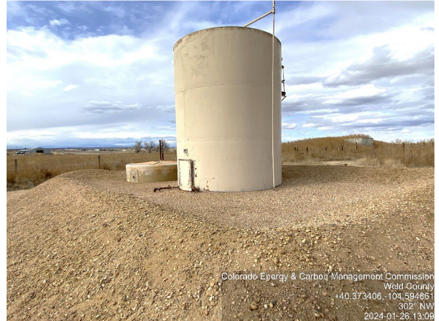
Photo #2 Lion #2 Battery site Active Tank(s): SE corner
