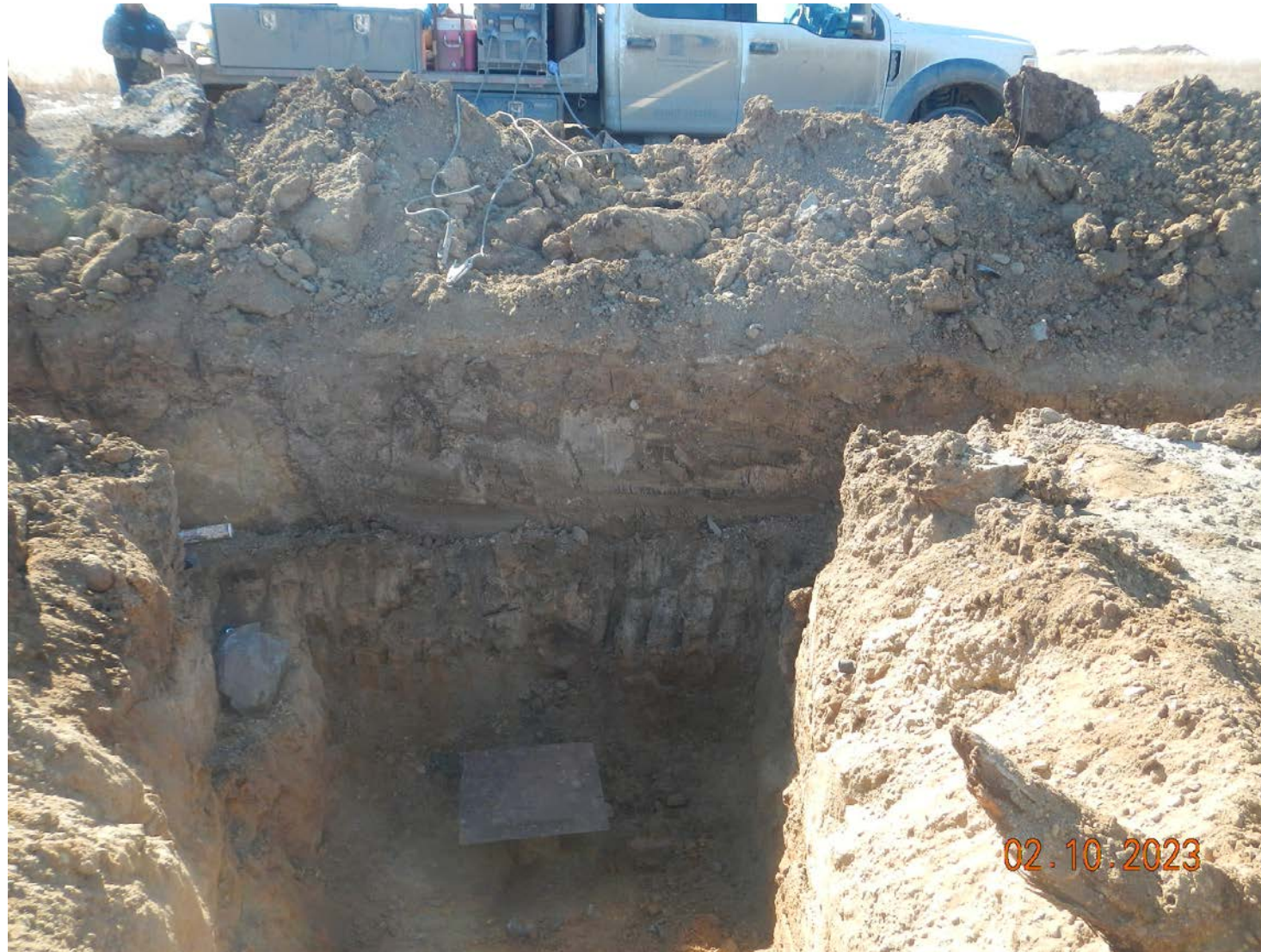
• Photo 2 – Wellhead view south
