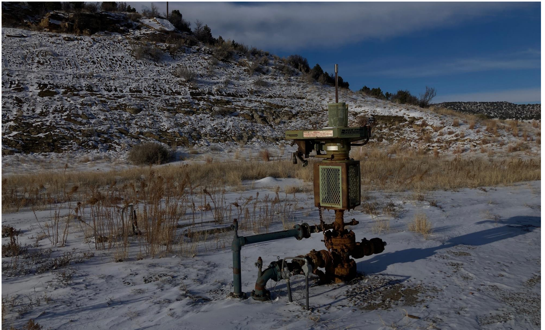
PHOTO 3: WELLHEAD AND EQUIPMENT
