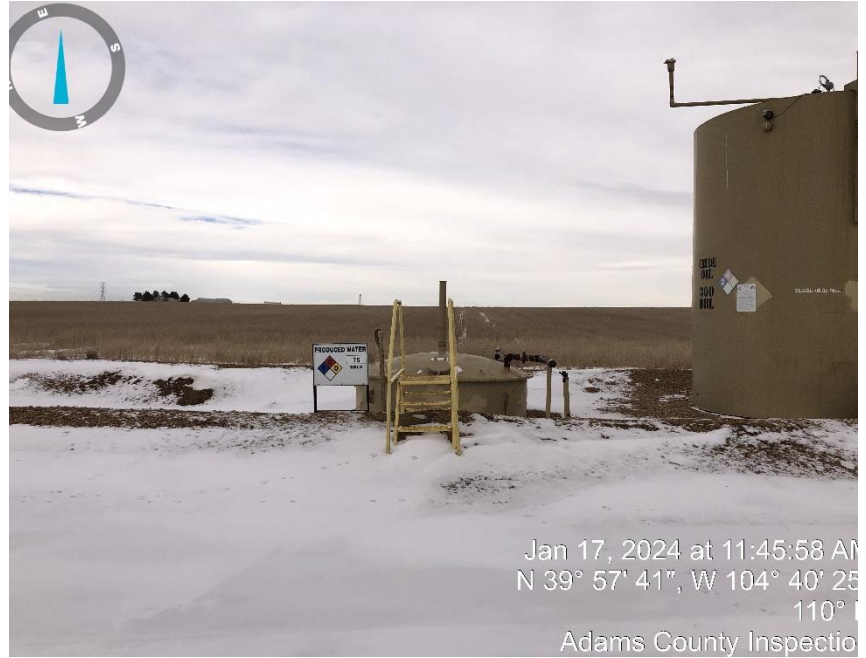
Photo #2 P/W tank.
