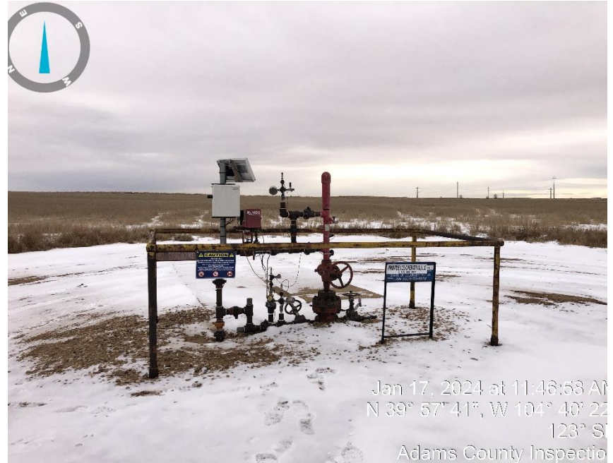
Photo #4 Well head.
