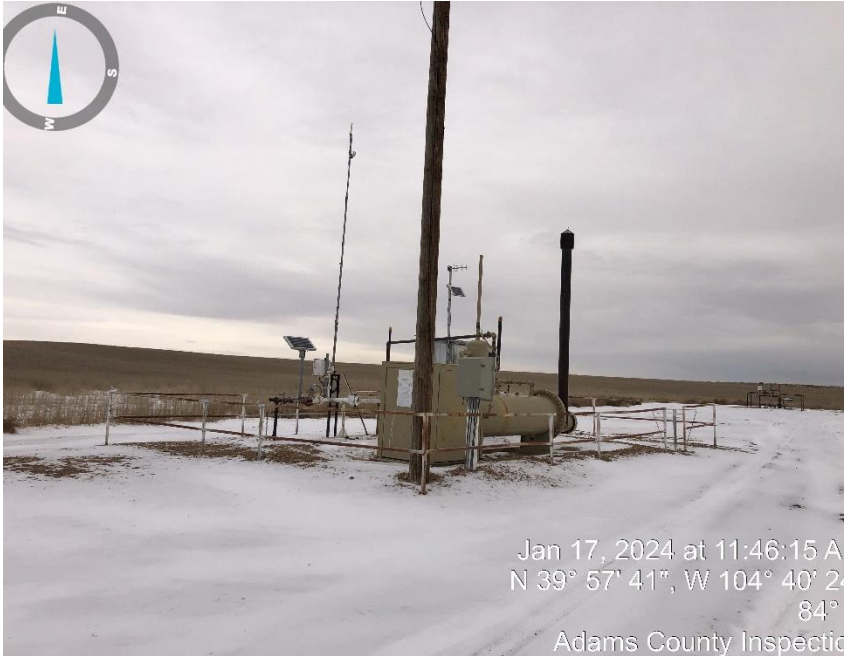
Photo #3 Meter & Separator.
